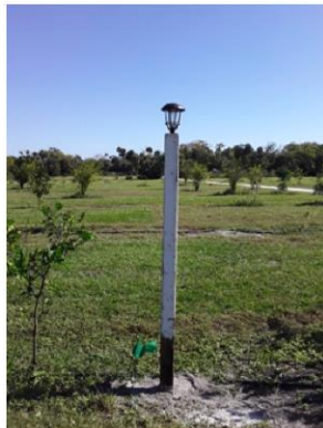
Solar Lighting to assist guests to their cars
